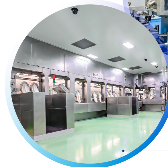
Injectable Filling Line
